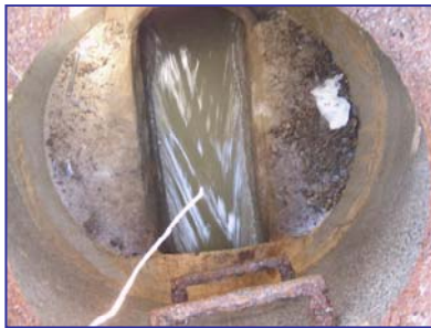
Flow measurements are taken throughout the collection system to determine the correct pump station upgrade size.
