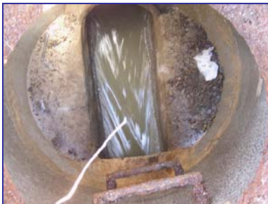
Flow measurements are taken throughout the collection system to determine the correct pipeline size.
