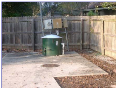
Pump Station #336, located on Nicholson Road, near Riverbend Road, will be upgraded.
