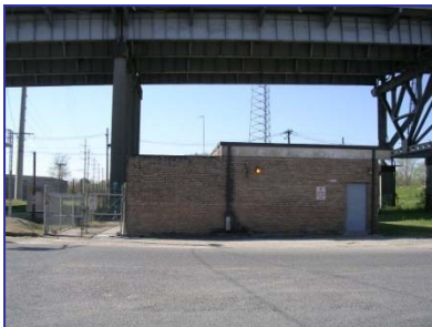
Pump Station 59 was upgraded from 7,777 GPM flow to a peak wet weather flow of 26,600 GPM.
